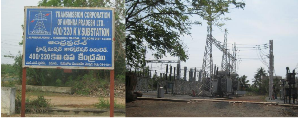
Figure 2.14 Electrical Substation near Manubolu
